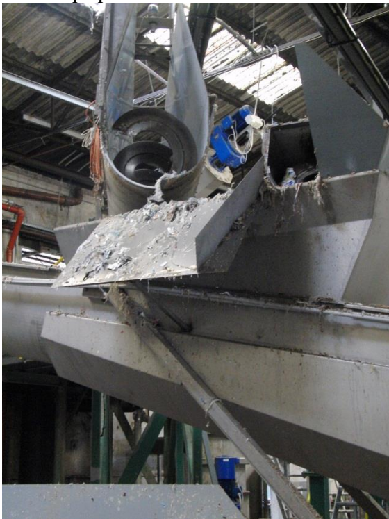
Figure 42: Screw feeders in the recycling plant.
